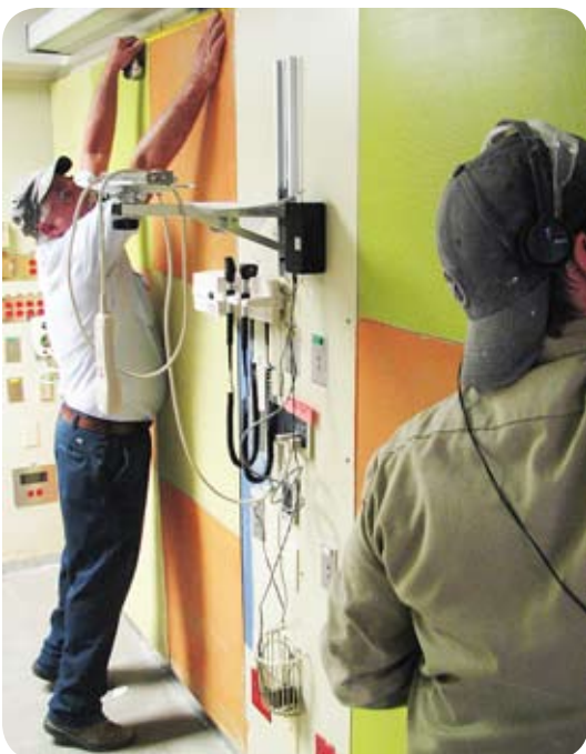
Shands Facilities construction workers are busy completing the patient rooms for the Pediatric Hematology/Oncology Immunocompromised Unit.
